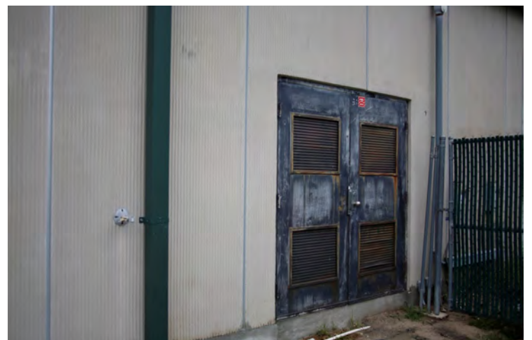
Mechanical room in need of upgrade
