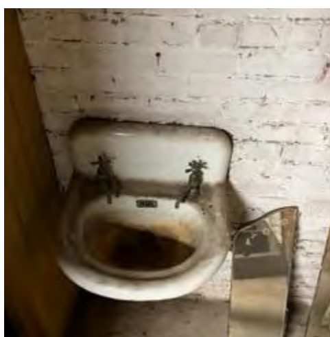
Old, unusable fixtures in basement
