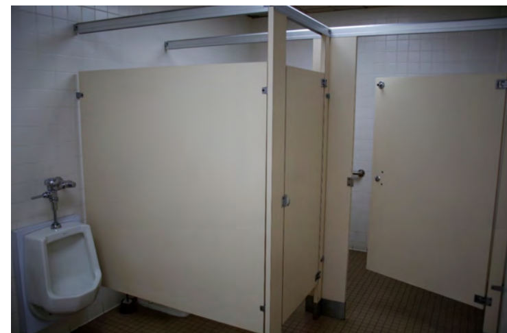
Restrooms difficult to navigate, not fully ADA compliant
