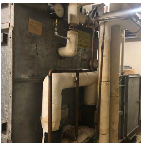
Sorely outdated HVAC
