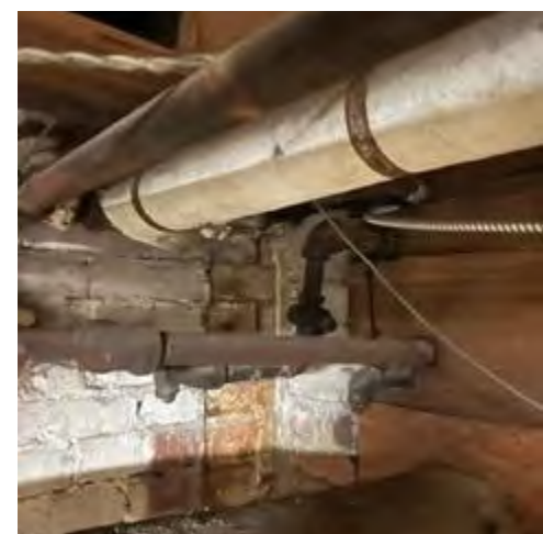
Failing structural integrity
