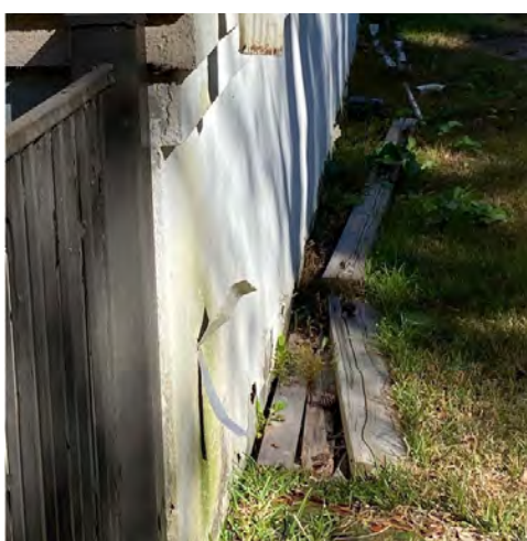
Bulging & cracking in the foundation
