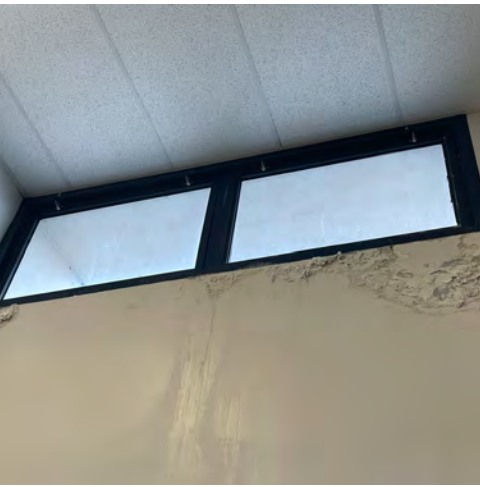
Deterioration around windows
