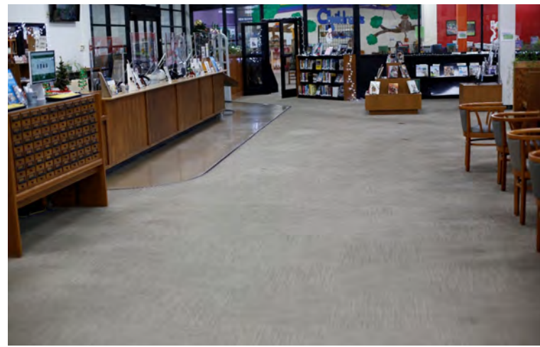
Worn, outdated interior
