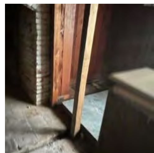
Basement in need of proper structural support
